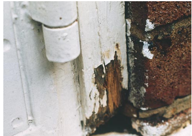
Figure 3: Wet rot decay in window joinery due to poor detailing between the sill and brickwork
