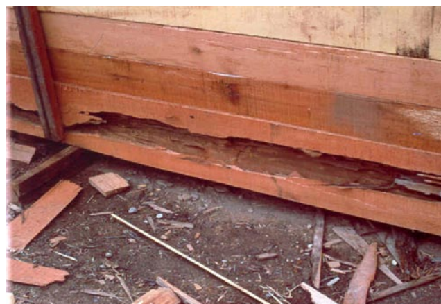
Figure 6: Termite attack in building timbers
