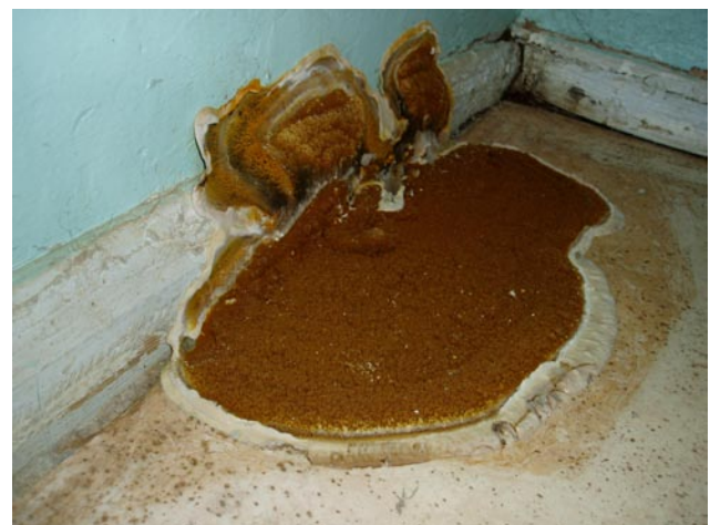
Figure 4: Dry rot attack in building
