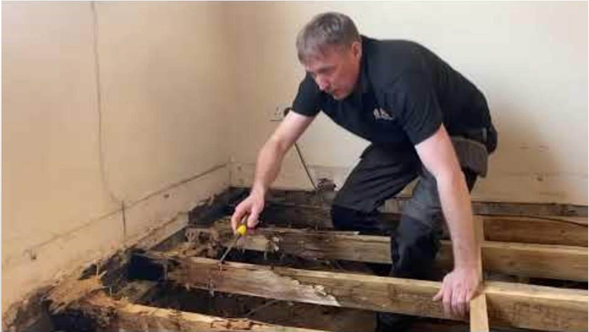
Wet Rot In Joists 4.48m
