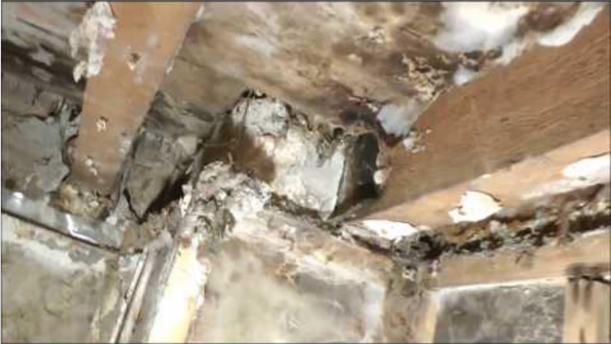
Dry Rot Out Break 4.48m
