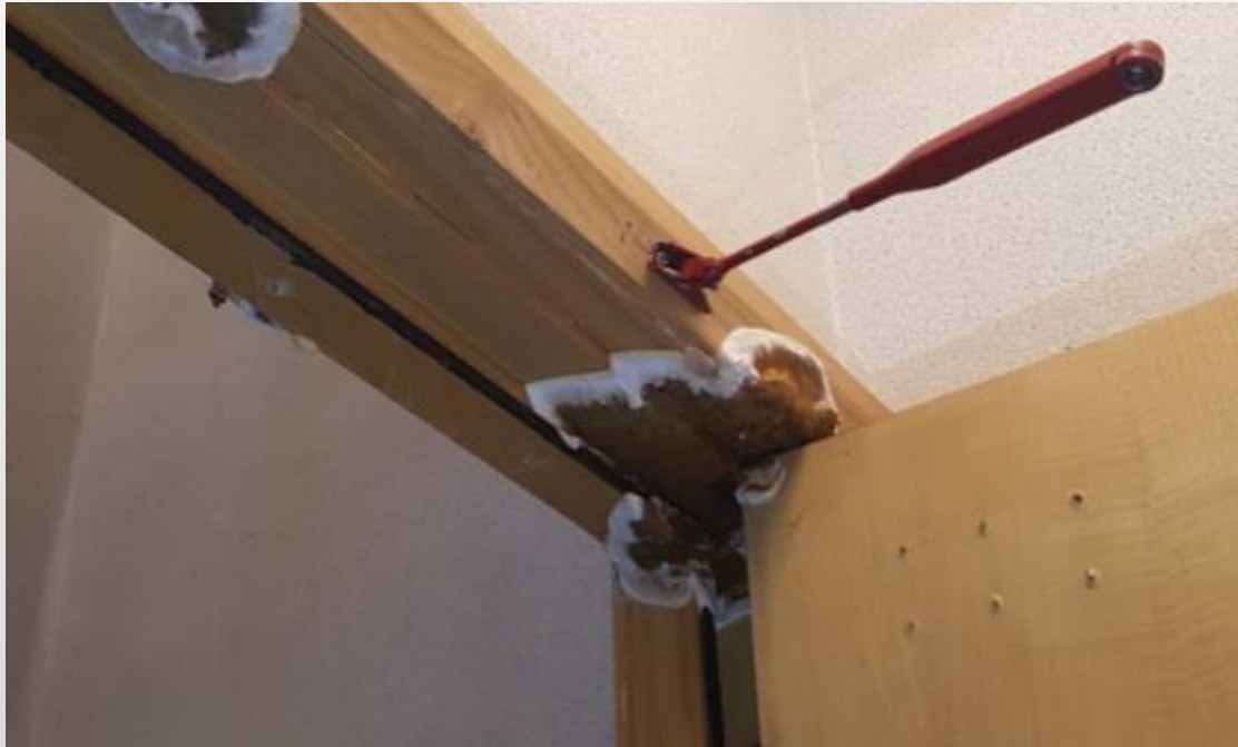
Dry Rot on internal door jamb.
